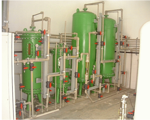
Figure 3. Water treatment located outside the reactor building.
