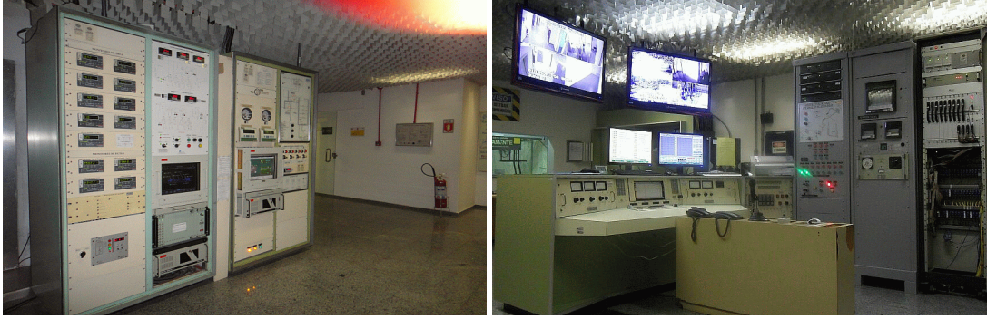
Figure 7. Reactor control room, radiation monitoring, pumps vibration monitoring and SVAC system (left). Control console with data acquisition system and CCTV surveillance (right).
