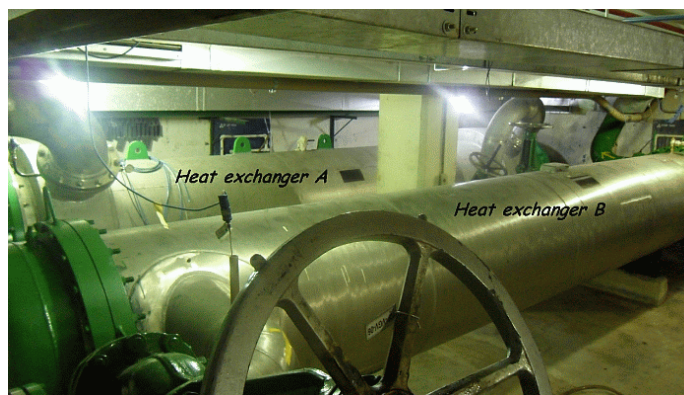
Figure 5. Heat exchangers A and B located in the reactor basement.
