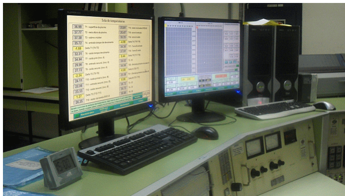
Figure 6. Data acquisition system in the control room.
