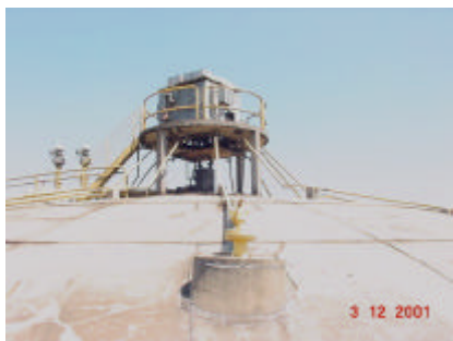
Figura 1 (a): Cúpula do digestor (L.C. Helou)
