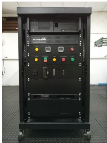
Figure 5: The control cabinet of the IFAC.
