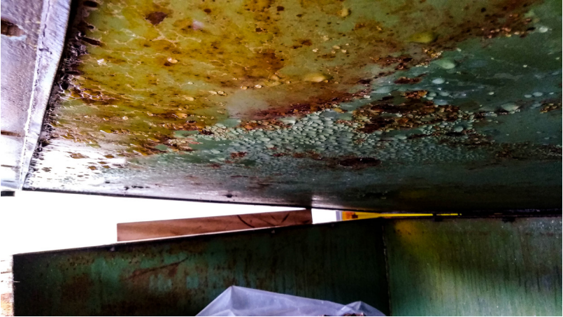
Figure 2 - Inside of the box that showed the highest moisture content. Note the water droplets formed by condensation in the underside of the box lid.
