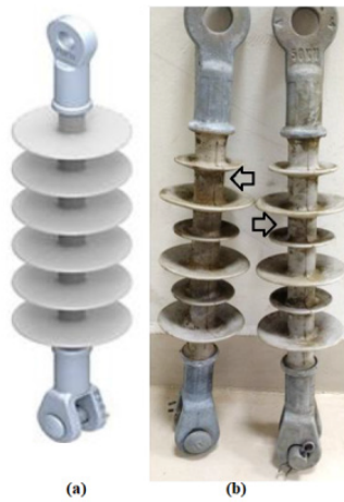
Fig. 1. Rod insulators based on SiR commonly applied to high-voltage (15 kV) power line to support conductor and insulate from ground (a) before use and (b) after nearly five years in operation at the altitude of 850 m, temperate climate with annual rainfall precipitation of 1375 mm, and average temperature of 21 °C in the region of Itajubá, Minas Gerais-Brazil. The arrows indicate some of the points of the insulator colonized by microorganism Trichoderma spp.
