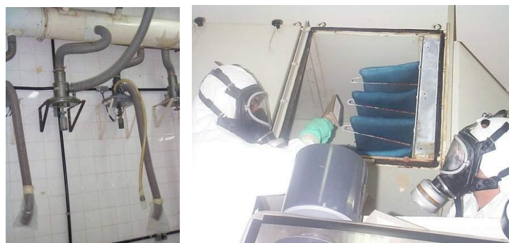
Figure 11. Exhausting system dismantling (left) and monitoring of the exhausting system absolute filters (right).
