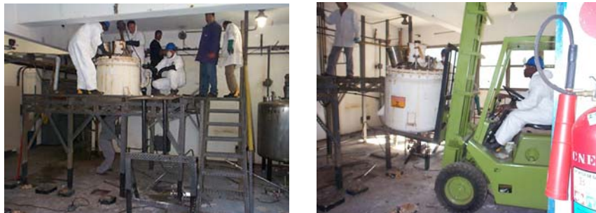
Figure 1: The removal operations of the impure yellow cake dissolution reactor.
