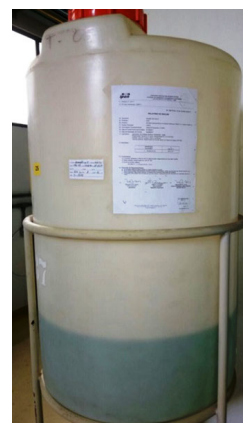
Fig. 1. UF 4 effluent tank at the installation
