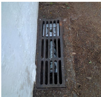
Fig. 2. Integrated collector installed in the street
