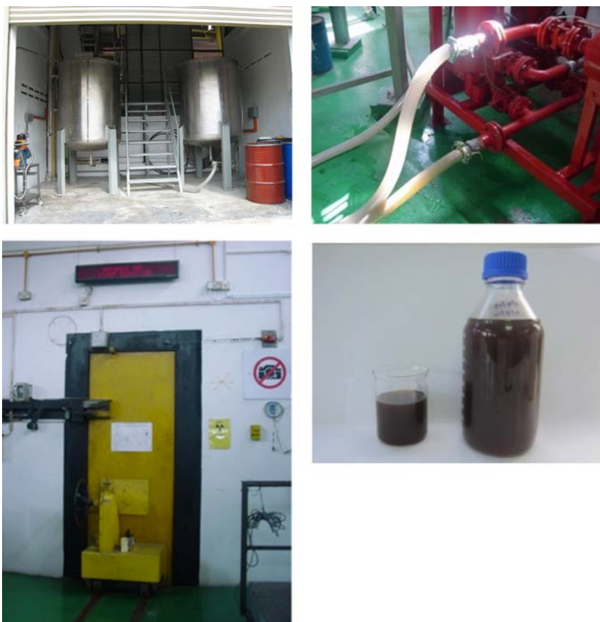
FIG. 8.14. Mixing and storage tanks (top left), pumping system (top right), irradiation room (bottom left) at the gamma irradiation pilot plant facility for continuous production of oligochitosan (bottom right), 2000 m 3 per cycle, in Malaysia.
