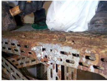
Figure 4: Corrosion observed in some perforated carbon steel structures after more than a decade since the interruption of the activities.
