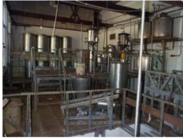
Figure 1: Third level of the Uranium Purification Pilot Plant, assembled with perforated steel structures.
